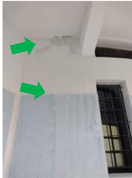
Figure 2 - Moisture stain present on the west façade.
