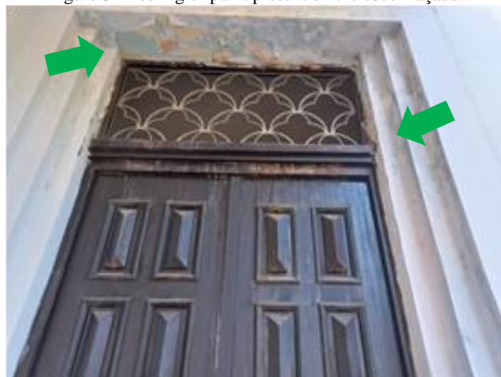
Figure 3 - Peeling of paint present on the south façade.
