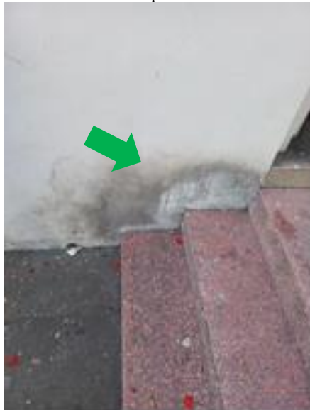
Figure 1 - Efflorescence present in the south façade.
