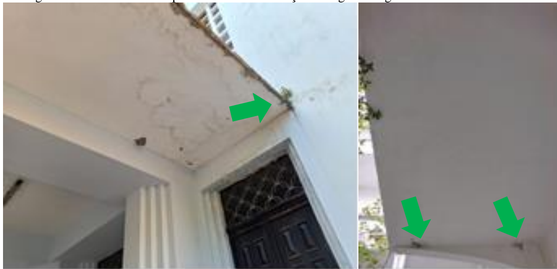
Figure 4 - Biodeterioration present in the south façade. Vegetation growth B. Presence of Mold
