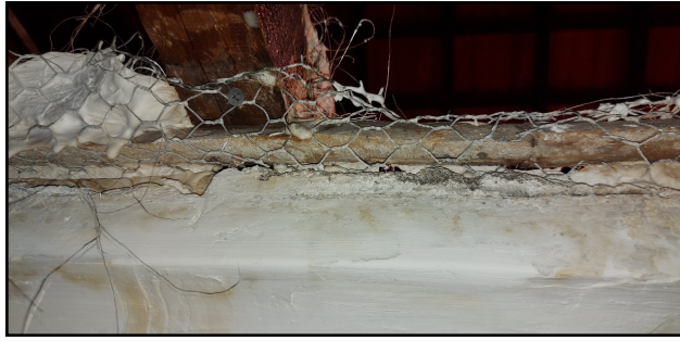
Figure 10 – Photo of the metallic mesh found between the lath and the cladding layers on the ceiling of the São Bento train station.
