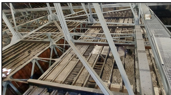
Figure 12 – Wooden elements in rectangular cut and use of new materials, present in the structure of the stucco ceiling of the São Bento station.
