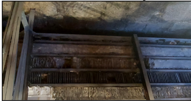
Figure 6 – Photo of the wooden structure of the stucco ceiling of the São Bento train station.
