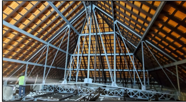
Figure 2 – Photo of the lattice metallic scissors with Pratt typology on the roof of the São Bento train station.
