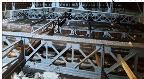
Figure 7 – Photo of the metallic structure of the stucco ceiling of the São Bento train station.
