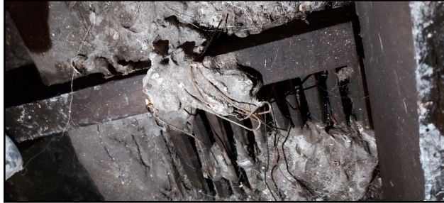
Figure 11 – Photo of the wires on the roof of the São Bento train station.
