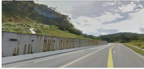
Figure 11. Containment structure - bolted curtain.
