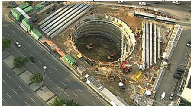
Figure 3: Praça da Bandeira Detention Reservoir (under construction), Rio de Janeiro – RJ – Adapted.
