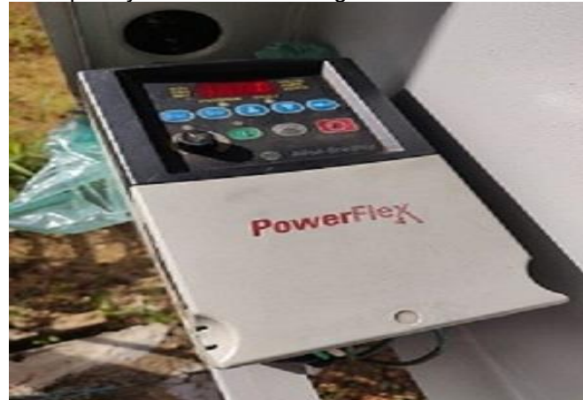
Figure 4 - Frequency inverter used to regulate the rotation of the fan rotor
