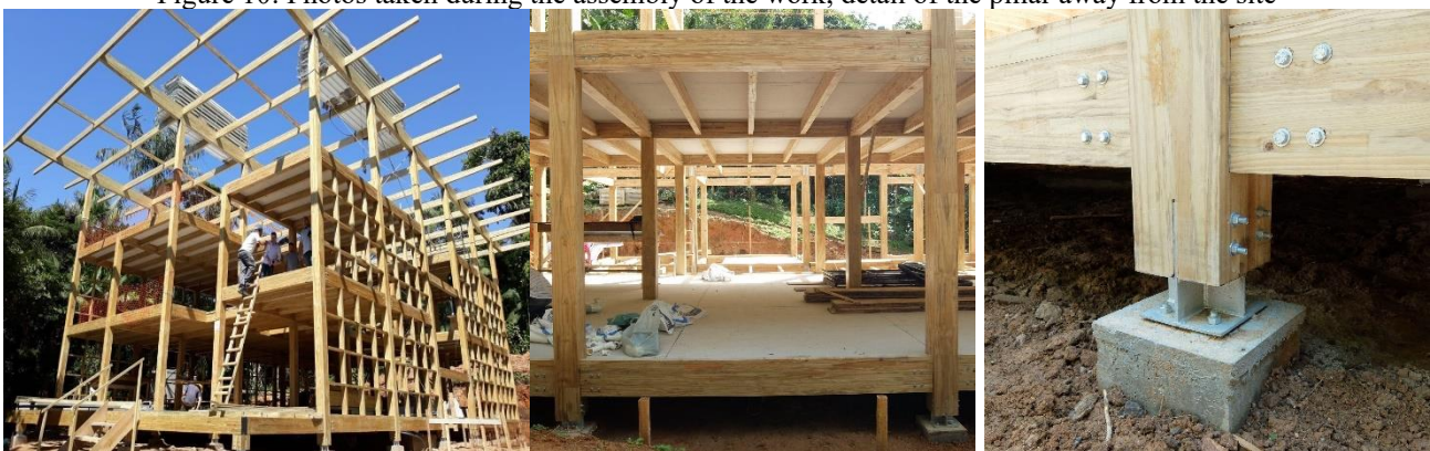
Figures 8 and 9: Photos taken during the assembly of the work, shows the grid structure of the MLC Figure 10: Photos taken during the assembly of the work, detail of the pillar away from the site
