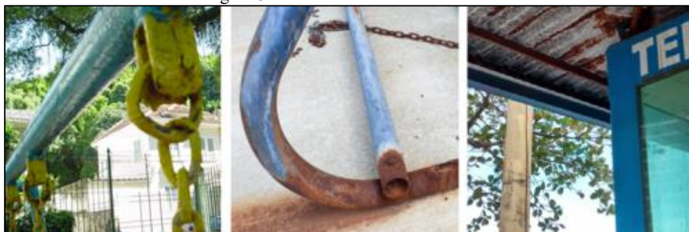
Figure 3 – Corrosion on street furniture
