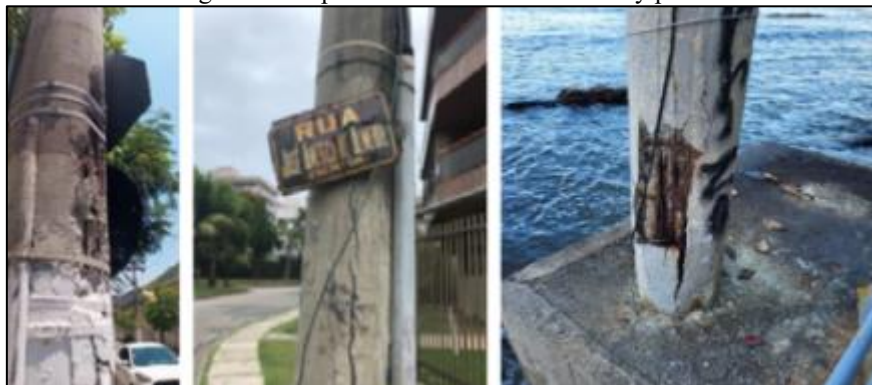
Figure 1 – Aspect of corrosion on electricity poles
