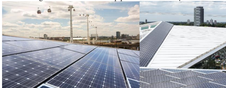
Figures 11 and 12: Rooftop photovoltaic solar panels
