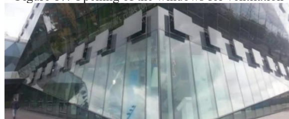
Figure 17. Opening of the windows for ventilation
