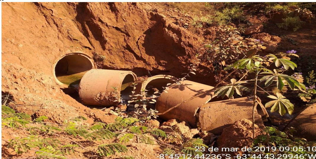
Figure 11: Culvert with a 1.50m shackle, where silting and silting problems were found. Erosive processes downstream of the channel
