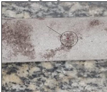
Figure 5 - Damage caused, holes going through the entire thickness. Source: The author.
