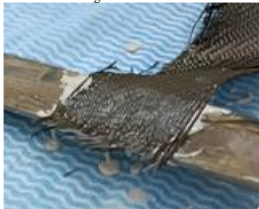
Figure 6 - Application of the adhesive together with the carbon fiber. Source: The author, 2023.
