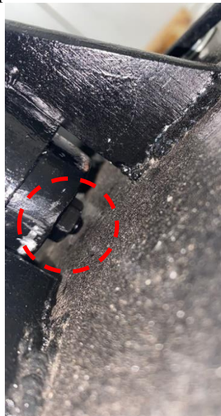
Figure 18 – Screw responsible for the rotation of the solar tracker structure.
