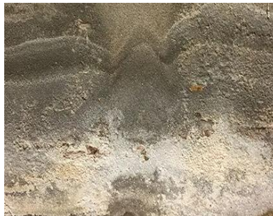
Efflorescence. Source: Aecweb (2023)
