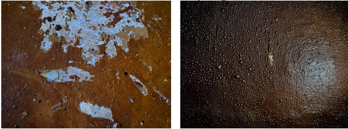
Figure 11 – Deterioration in the waterproofing of the reservoir
