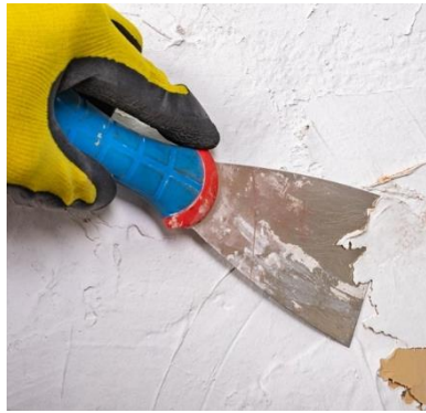
Paint deterioration – scraping. Source: Revprol (2022)
