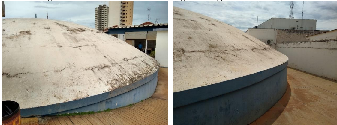
Figure 6 - Cracks and fissures located throughout the upper slab of the reservoir.
