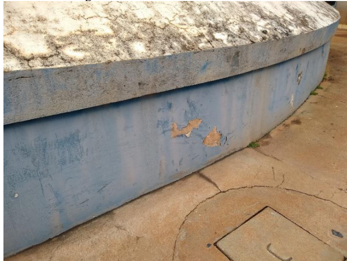
Figure 7 – Paint wear and deterioration
