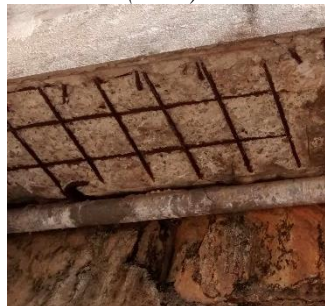
Corrosion in the armor Source: Silva (2018)
