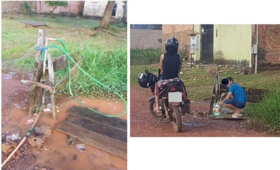
Figure 11 – Record of people taking treated water for human consumption in the pipe supplied by the general network
