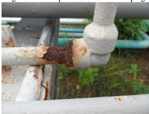
Figure 1: Atmospheric Corrosion in Piping.
