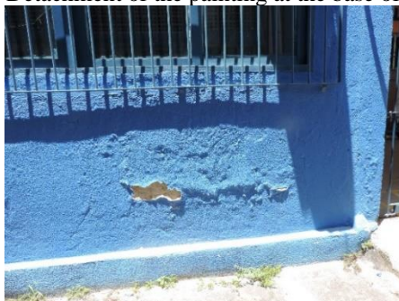
Figure 4 - Detachment of the painting at the base of the façade
