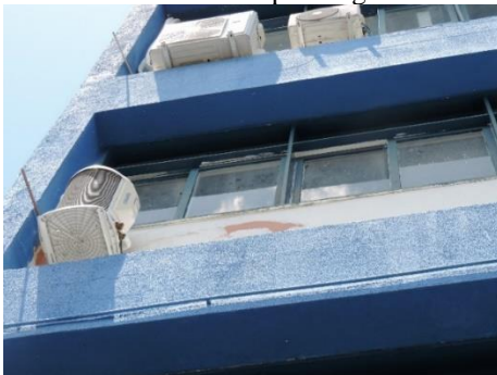
Figure 5 - Detachment of the painting near the windows
