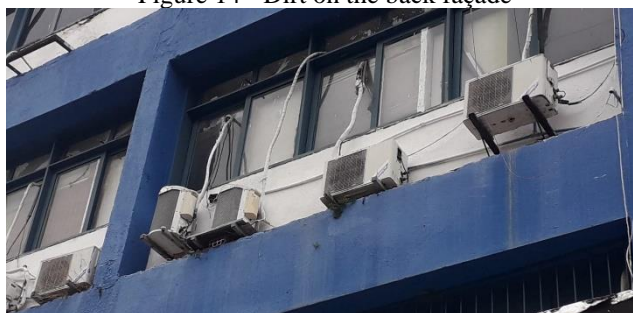
Figure 14 - Dirt on the back façade
