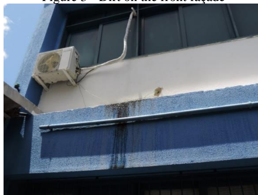
Figure 3 - Dirt on the front façade
