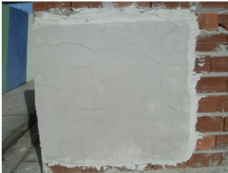
Figure 11: Formation of cracks mapped in direct application on masonry Source: ALVES JÚNIOR, 2009.
