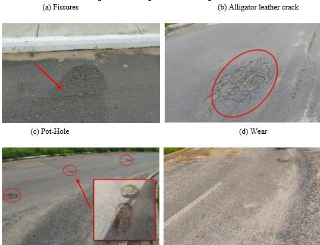
Figure 5. Pathologies observed in segment 1.
