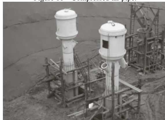
Figure 10 – Compressed air pipe.
