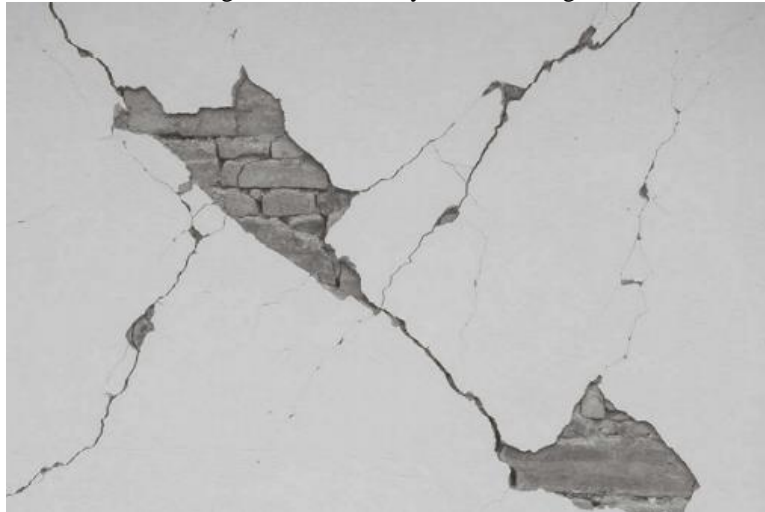
Figure 12 – Masonry with cracking.
