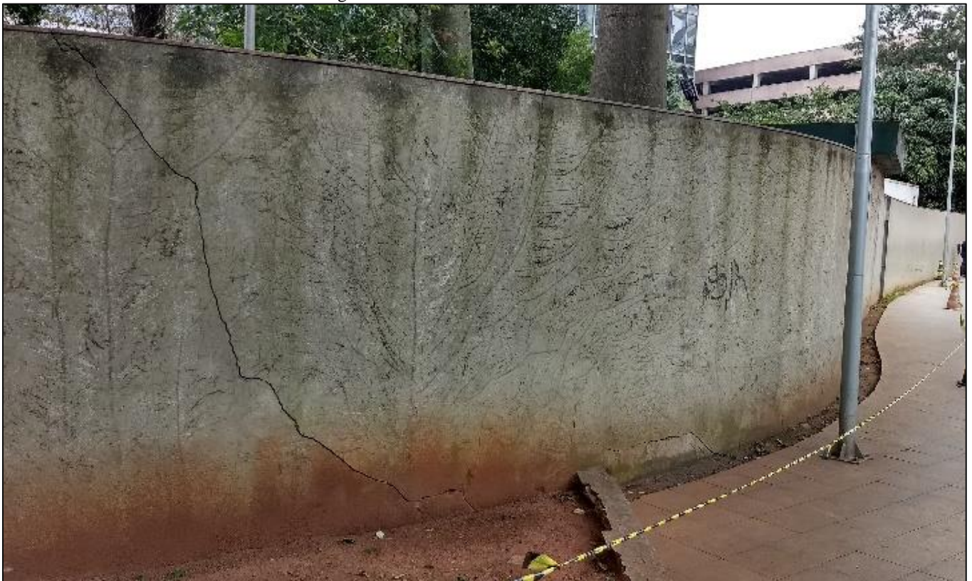
Figure 28 – View of the Crack in the Wall.
