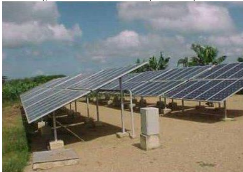
Figure 2. Santa María del Lotero photovoltaic plant.
