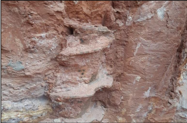
Figure 14. Continuous auger bit lost during pile drilling and found in the excavation underground.
